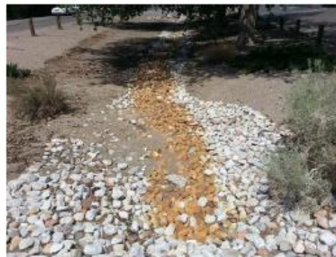
Dark staining in waterway
