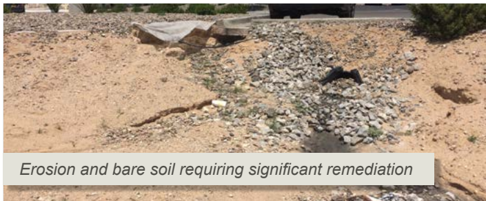
Basin clogged with sediment no longer infiltrates water
