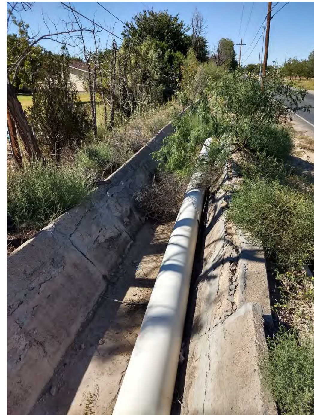
Figure 6.5.1 Pressure Piped Elephant Butte Irrigation District Facility
