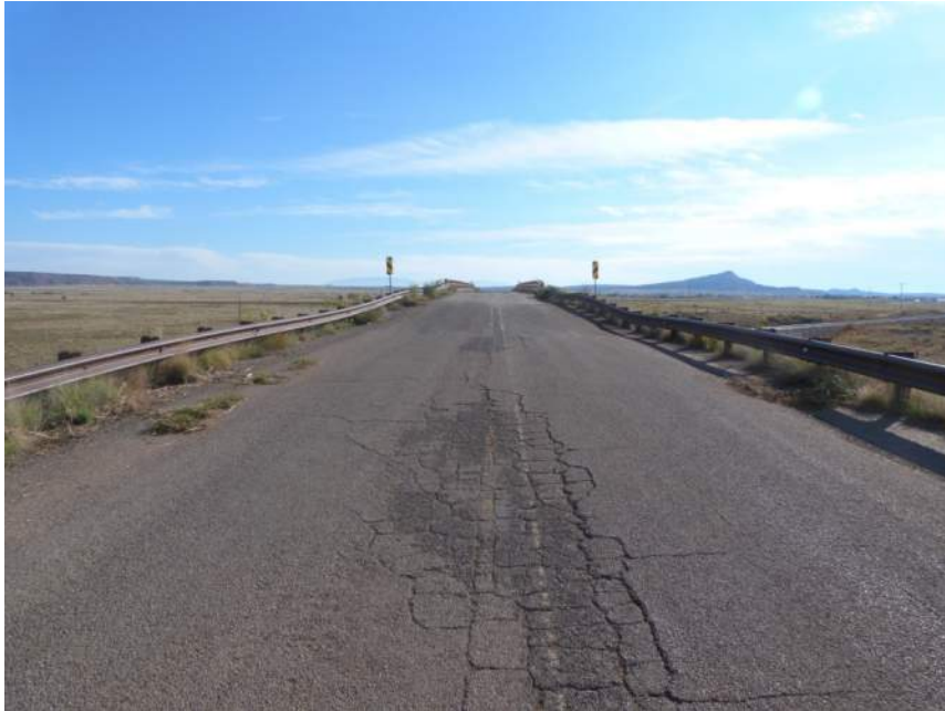
Figure 4. Wide/Deep Lateral and Transverse Pavement Surface Cracking (Alligator Cracking)
