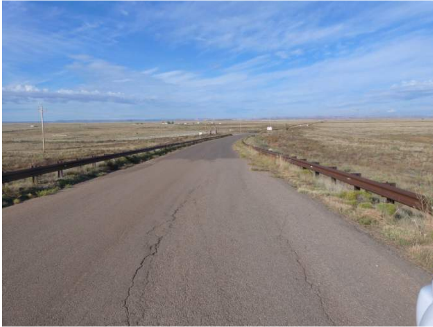
Figure 6. Lateral Cracking and Deterioration of Pavement Shoulder (Vegetative Overgrowth/Encroachment)
