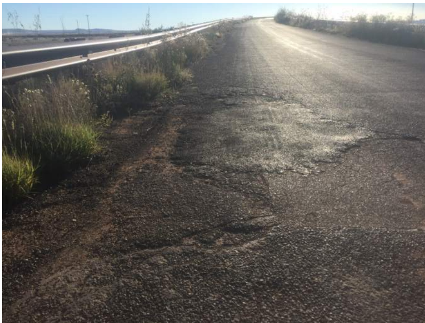
Figure 5. Exposed Base Course and Pavement Patching
